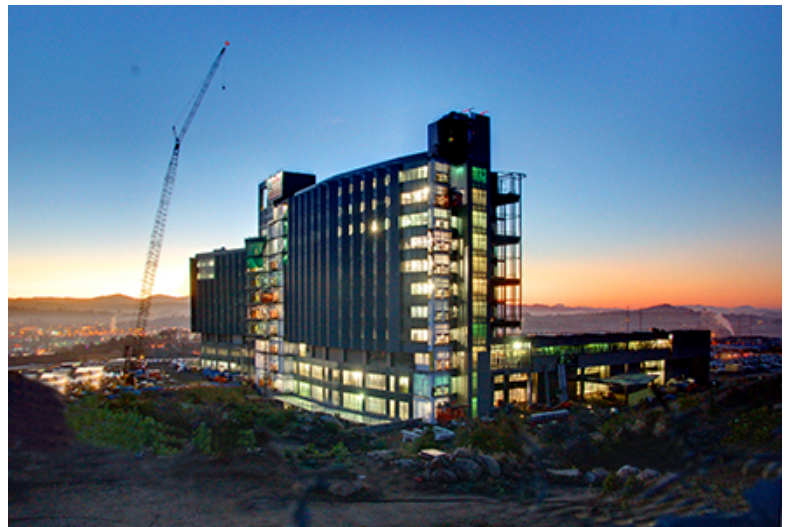
Palomar Medical Center West (PMCW) – DPR Construction Healthy Buildings is conducting mold and moisture monitoring during the construction phase of this major construction project
